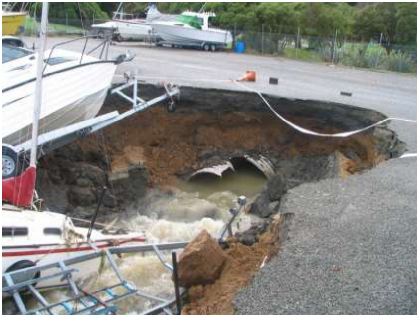
Figure 13 Collapse of area under the boat store 6 March 2014 storm
